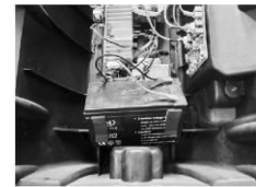
③ Take apart the battery wire
